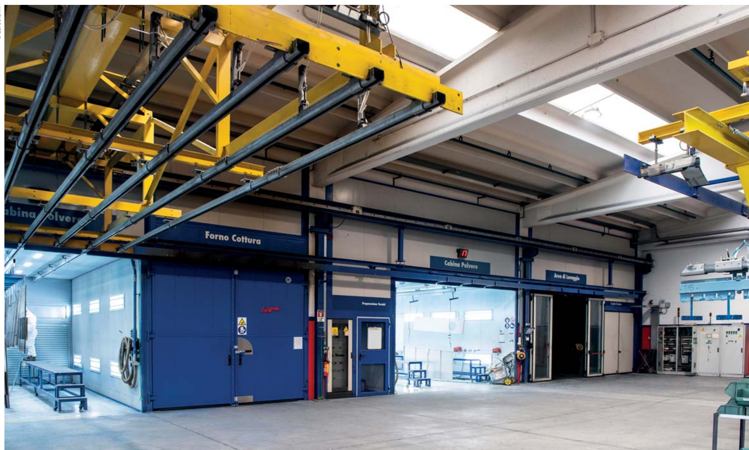
The coating department.
