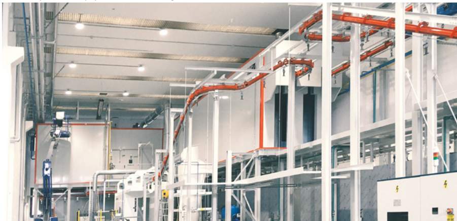
➤ Continuous powder coating system
